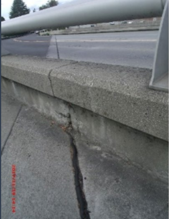
Expansion joint material on bridge containing > 4000 ppm PCBs Photo courtesy of BASMAA
