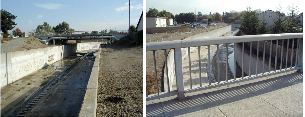
A) View looking upstream at the Washington Street Bridge. B) View looking upstream from the potential sample location on the upstream side of Washington Street.
