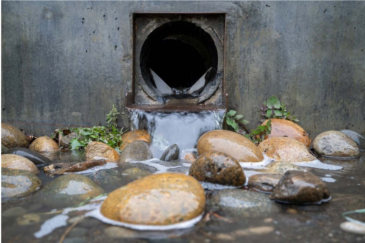
Figure 1: Storm flows into bioretention rain garden in San Francisco. Photo courtesy of Shira Bezalel.
