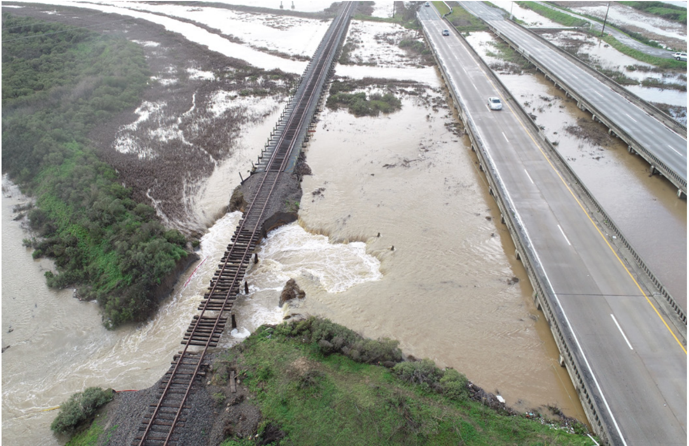
Flooding on February 14, 2019 damaged the SMART tracks just east of Novato Creek (creek channel visible in background). Photo by Marin County Department of Public Works.
