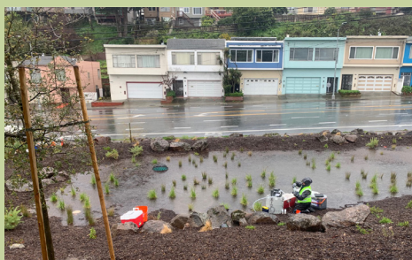
Rain gardens and GSI features (residential)
